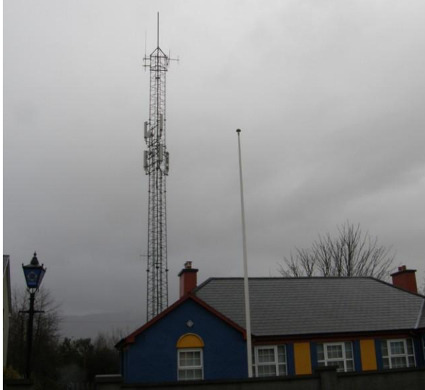
Transmitter Site Photo
